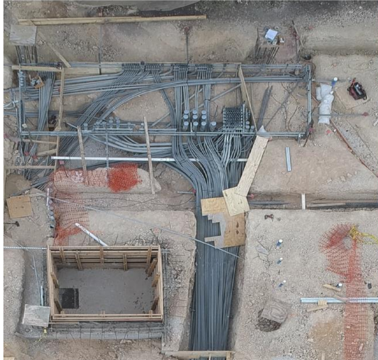
1st. Floor Underground - Electrical Duct Bank
